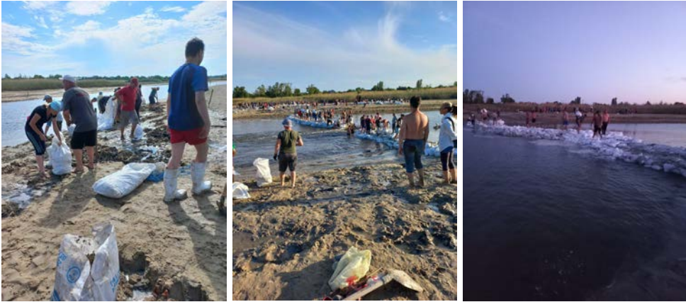
Construction of a self-improvised dam by locals, Kapulivka and Oleksiivka, Dnipropetrovsk Region, June 2023
